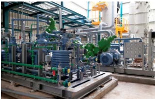
Figure 3. CPU general view Figura 3. Vista general de la CPU
